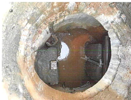
2#雨水排放口闸阀
