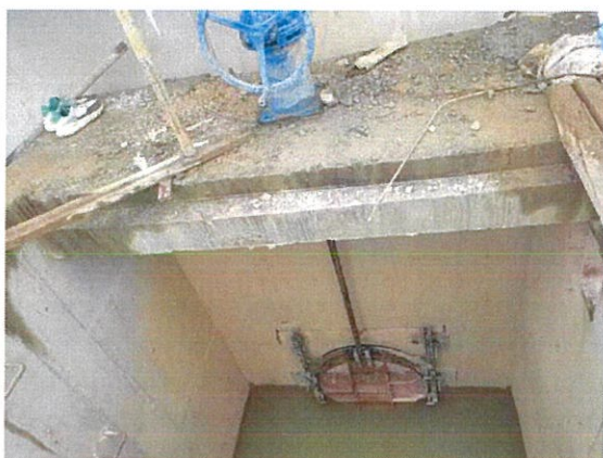
1#雨水排放口闸阀
