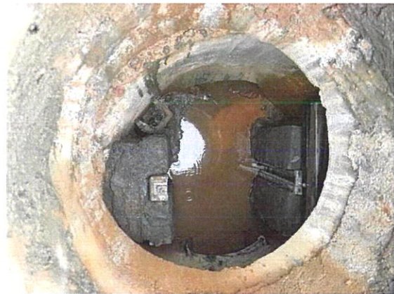
2#雨水排放口闸阀
