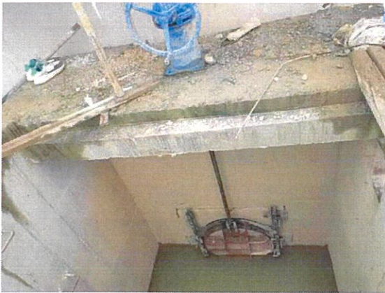
1#雨水排放口闸阀
