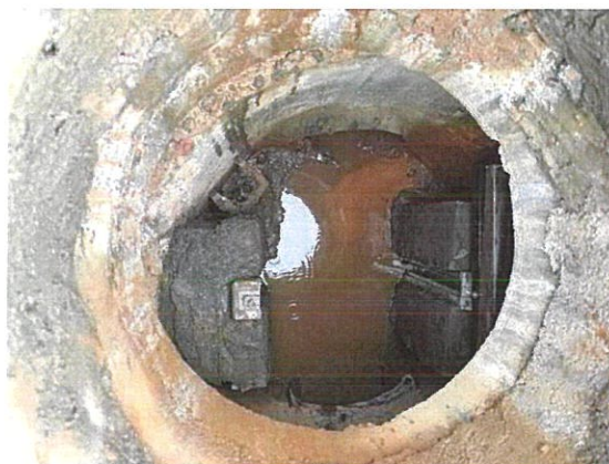
2#雨水排放口闸阀
