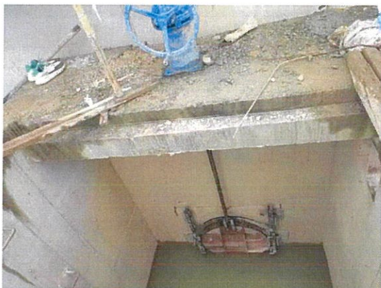
1#雨水排放口闸阀
